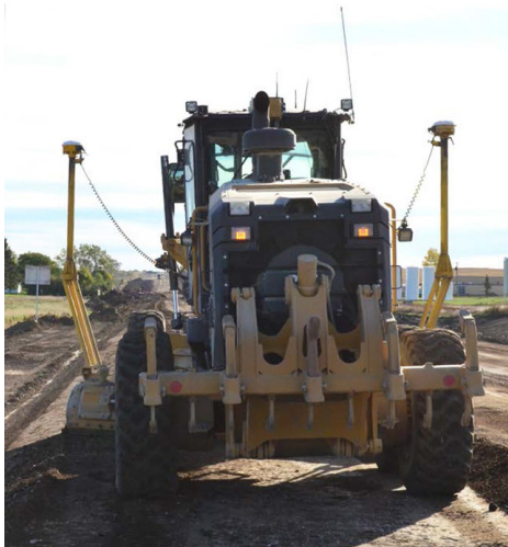
GPS-guided construction was just starting to take off when NCHRP Synthesis 372 assembled best practices on this and other new construction technologies.
